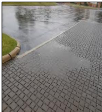
Surface ponding over PICP indicating clogged joints and the need for maintenance. Credit: Chagrin River Watershed Partners, Inc.
