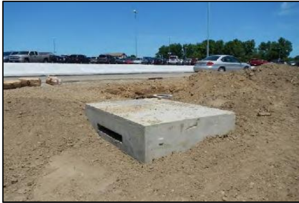
Sand filter installed to capture stormwater runoff from commercial parking lot . Credit: Ohio Department of Natural Resources Division of Soil & Water Resources.
