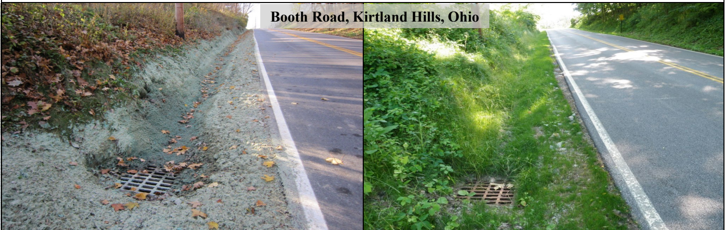
October 2011, Application of biostimulant additive with hydro mulch and ODOT Roadside Seed Mix
