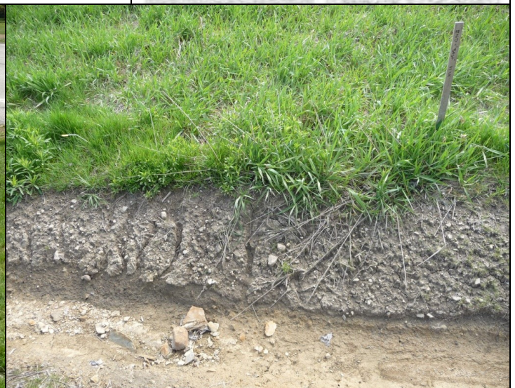
Standard hydro mulch application without biostimulant resulted in poor germination and rill erosion of the back slope
